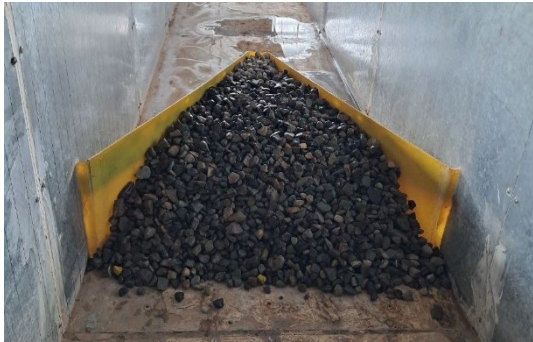
Fig. 4 A view of the sediment-filled state upstream of the spillway.
